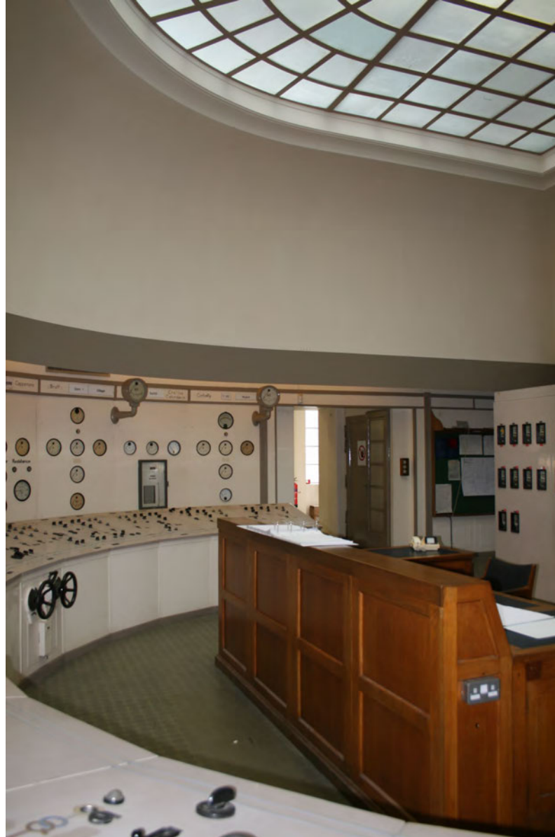
FIGURE 3-26 - ORIGINAL ARDNACRUSHA CONTROL ROOM SHOWING GLASS CEILING (PHOTOGRAPH TAKEN BY THE AUTHOR, AUGUST 2008)
