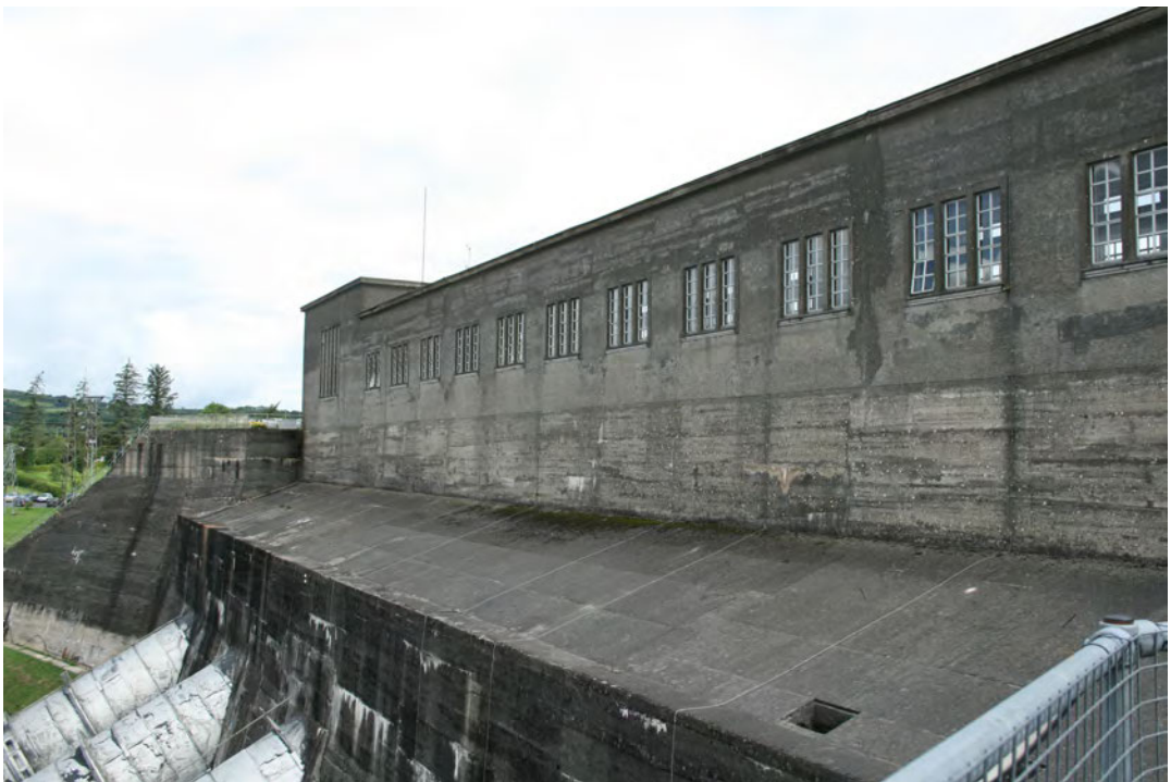
FIGURE 3-23 - SOUTH SIDE OF ARDNACRUSHA INTAKE BUILDING (PHOTOGRAPH TAKEN BY THE AUTHOR, AUGUST 2008)
