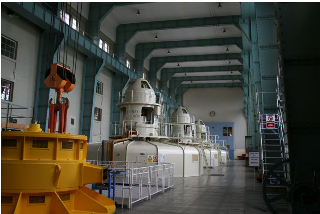
FIGURE 3-24 - INTERIOR OF ARDNACRUSHA TURBINE HALL (PHOTOGRAPH TAKEN BY THE AUTHOR, AUGUST 2008)
