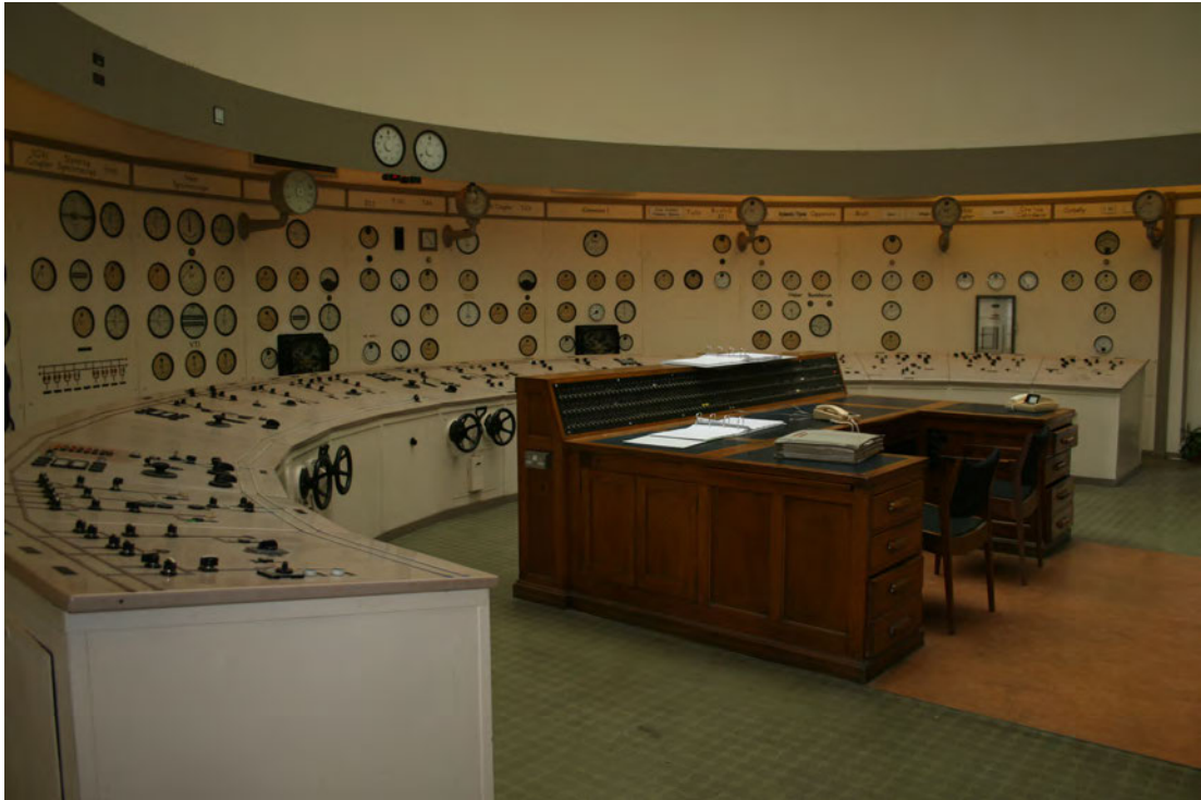
FIGURE 3-25 - ORIGINAL ARDNACRUSHA CONTROL ROOM (PHOTOGRAPH TAKEN BY THE AUTHOR, AUGUST 2008)
