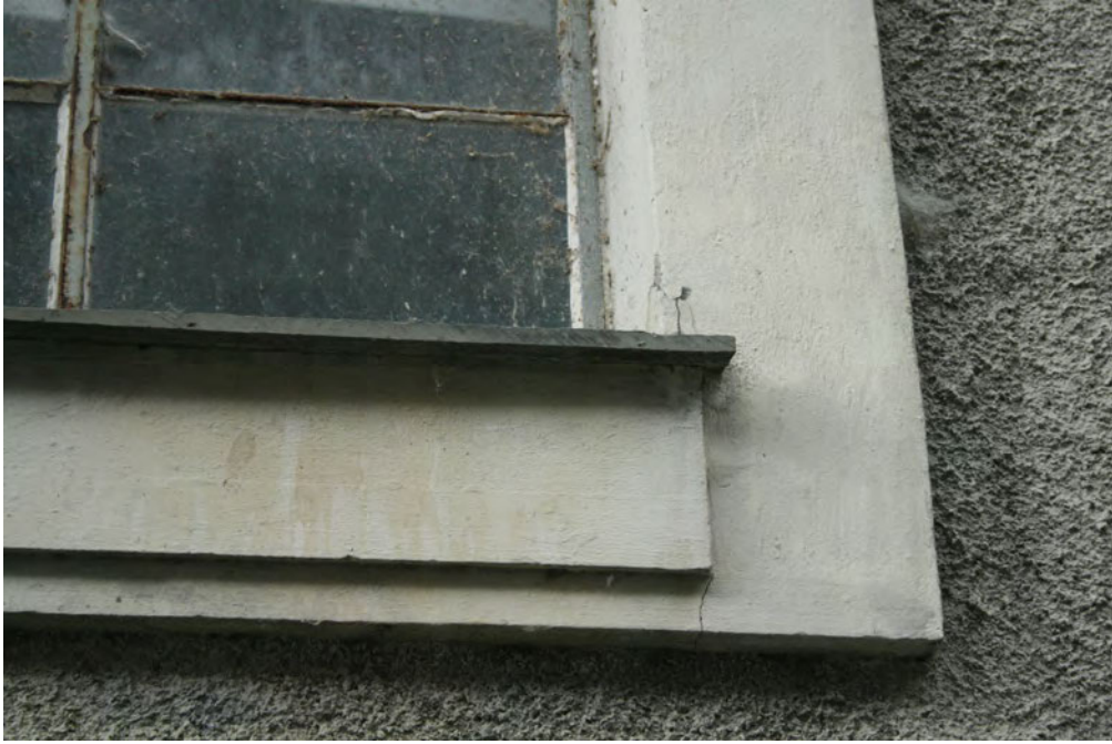
FIGURE 3-21 - DETAIL OF WINDOW FRAMES WITH ORIGINAL PAINTWORK, REAR OF ARDNACRUSHA POWER HOUSE (PHOTOGRAPH TAKEN BY THE AUTHOR, AUGUST 2008)
