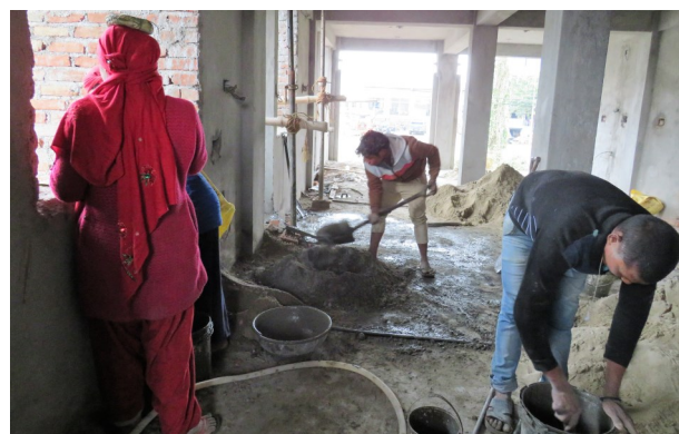
Young men and women are working in the house construction in urban Kapilvastu research site in Nepal
