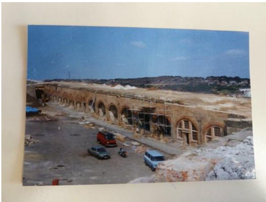
Fig. 3.10: Newhaven Fort being repaired, 1981, a view that Greg and Chris would recognise from living memory. Image: Newhaven Fort Archive.
