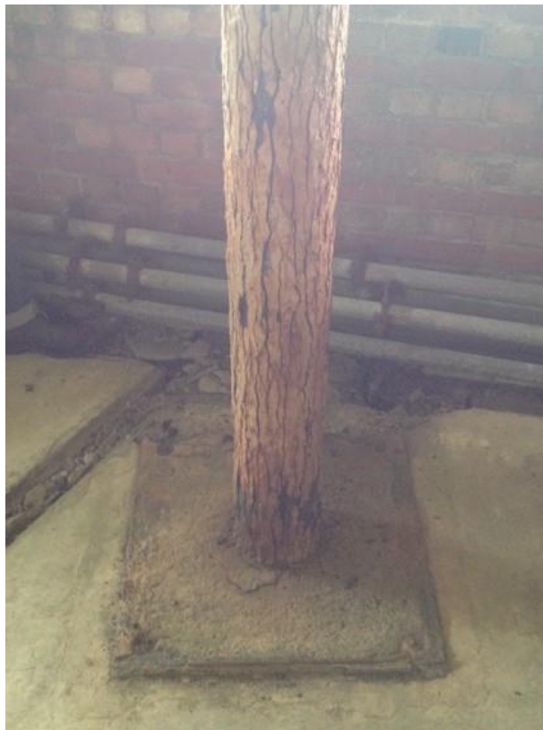
Fig. 7.24: Newhaven Fort, rusted support pole from southern lookout post to the English Channel, March 2018. Image: Harriet Parry.
