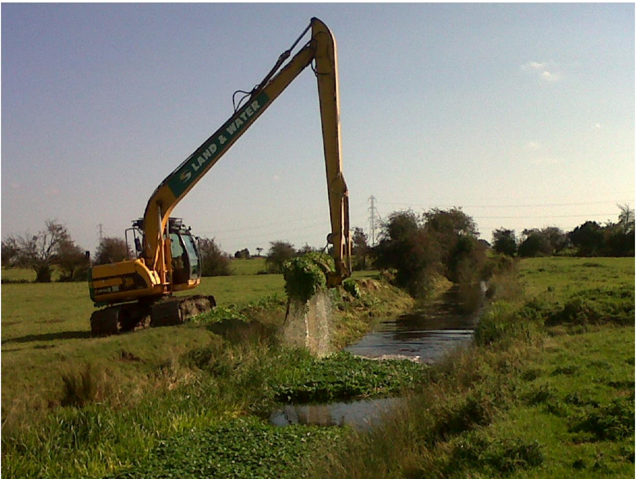
Figure 10: Example of excavator used for mechanical removal and de-silting, weed-cutting H. ranunculoides on the Pevensey Levels. (Photograph, Birch J).
